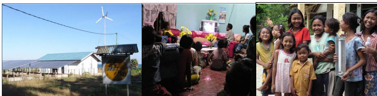
Figure 8. PVES introduction into a community should aim to increase RSC: 1) The PV-Wind-Diesel hybrid installation and PLD institution (physical capital and social capital). 2) Neighbors assembled to watch TV in Oeledo (social capital) and 3) Young villagers share the excitement of a new SHS installation in Lampung (social capital).
